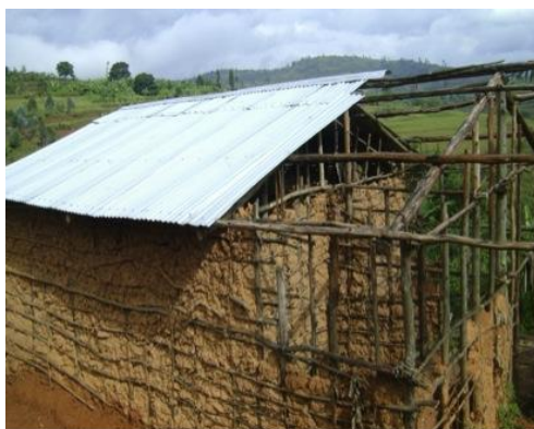
House being built for Alvera Mukankusi whose husband killed and house destroyed during genocide.
